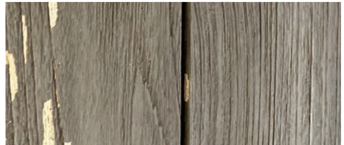
Partial weathering (some unpainted teak exposed)
