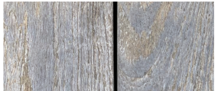
Advanced weathering (most finish worn away)
